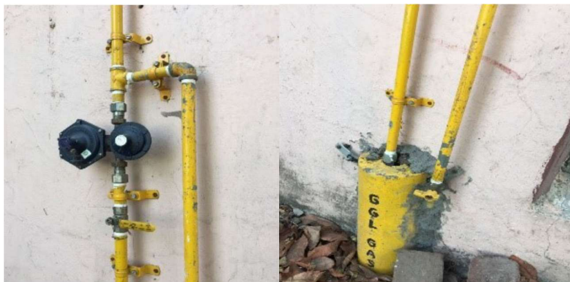
Figure-11: Stagnant riser pipelines and tapping points
